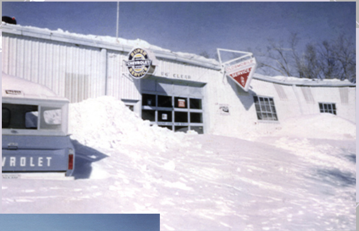
Heavy snow caved in the roof of a local car dealership in Buffalo during the Blizzard of '71 (photo courtesy of Joanne McVicker)
